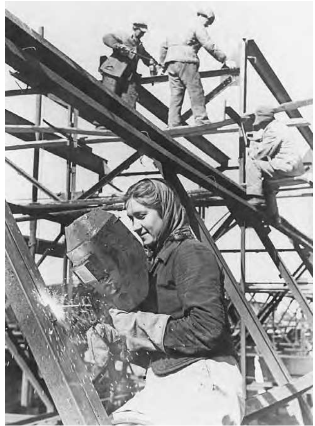
A woman welds beams at the site of a tractor factory in Belarus, 9 May 1947. The factory construction was part of the post-war Five-Year Plan. (Bettmann/Corbis)
