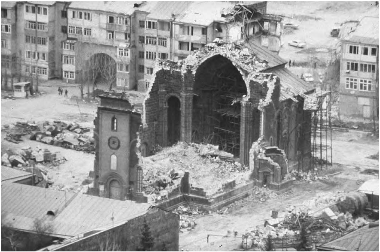
Collapse of an old stone masonry Armenian church in Leninakan, Armenia, following a catastrophic earthquake on 7 December 1988 that killed between 25,000 and 50,000 people. (C. J. Langer, U.S. Geological Survey)
